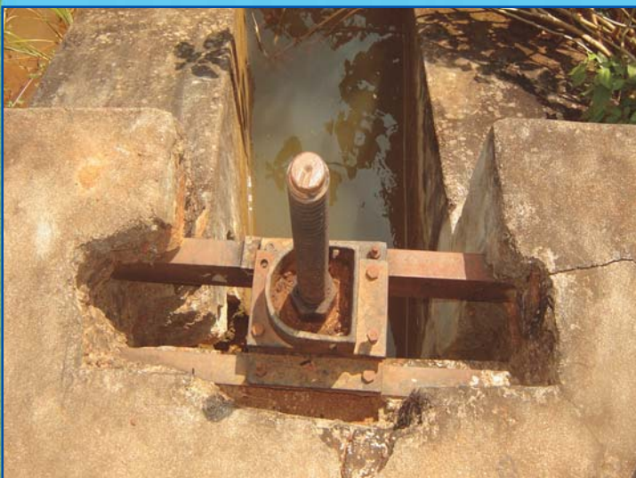
Damaged Sluice to be repaired under the Project
